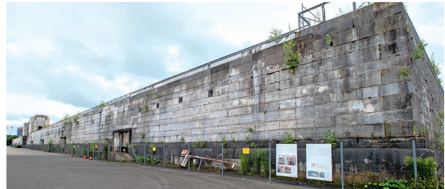
Fencing along the entire rear of the Grandstand protecting pedestrians against falling masonry.
