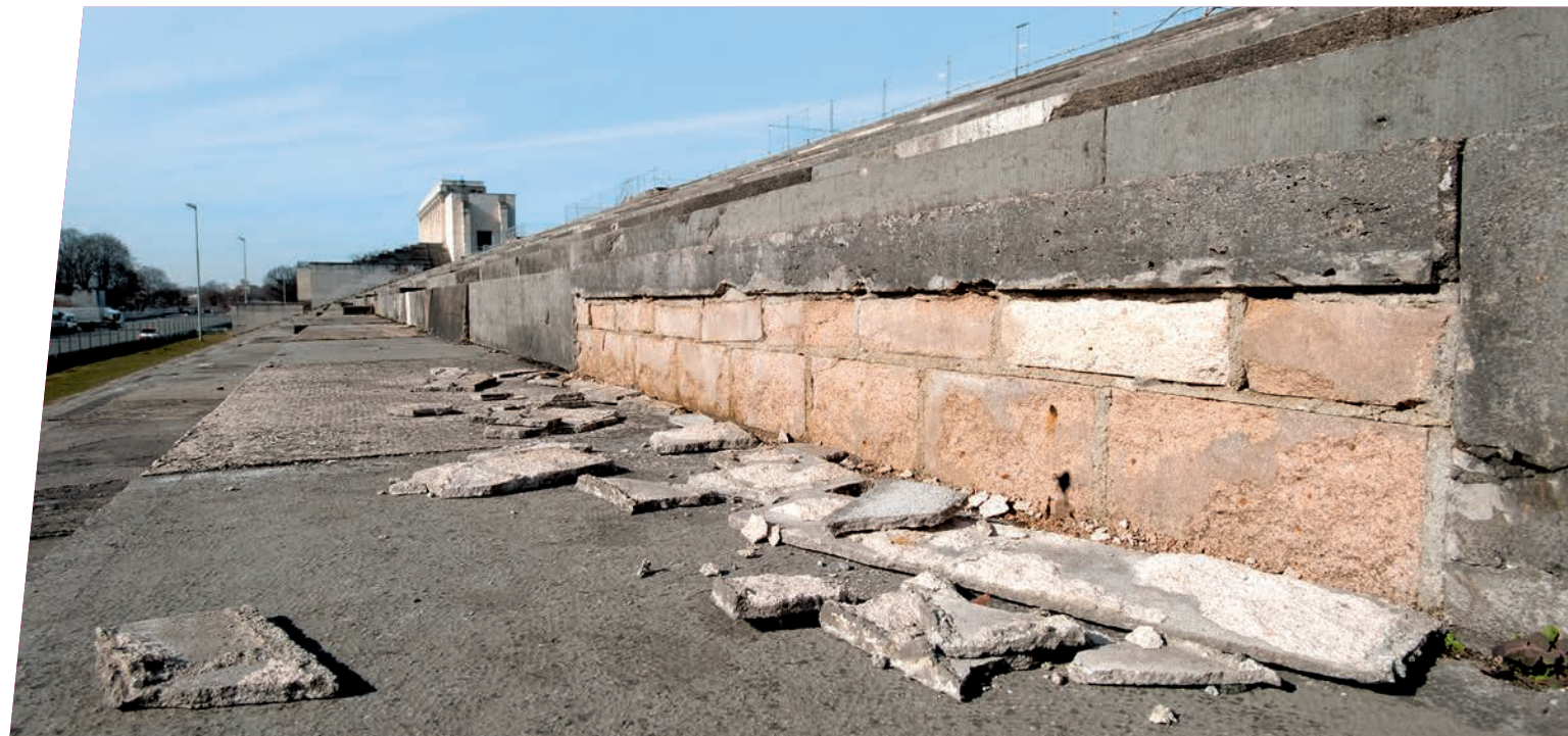
In many places, the facing of the steps on the Zeppelin Grandstand has collapsed.
