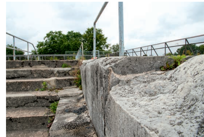
Everywhere split-off fragments of stone are conspicuous. Many blocks of stone are irreparably damaged.
