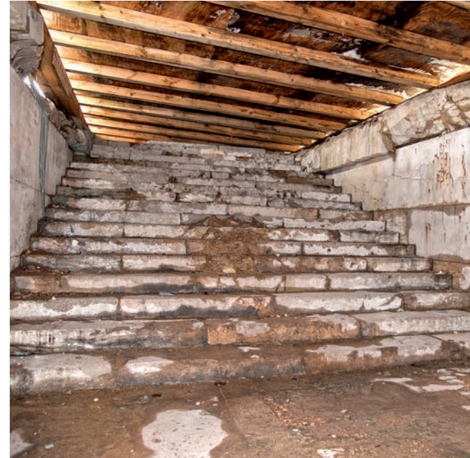
The interior stairwells in the Zeppelin Grandstand were temporarily closed off with wooden roofs.
