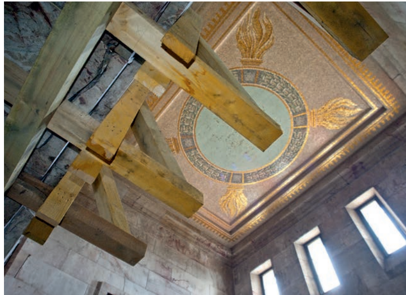
In many places in the Zeppelin Grandstand, wooden constructions are needed to support the ceilings.
